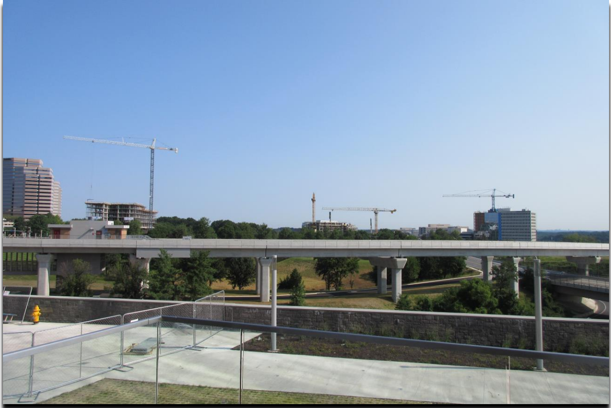
View of construction activity in Tysons from the base of Tysons Tower (July 30, 2014)
