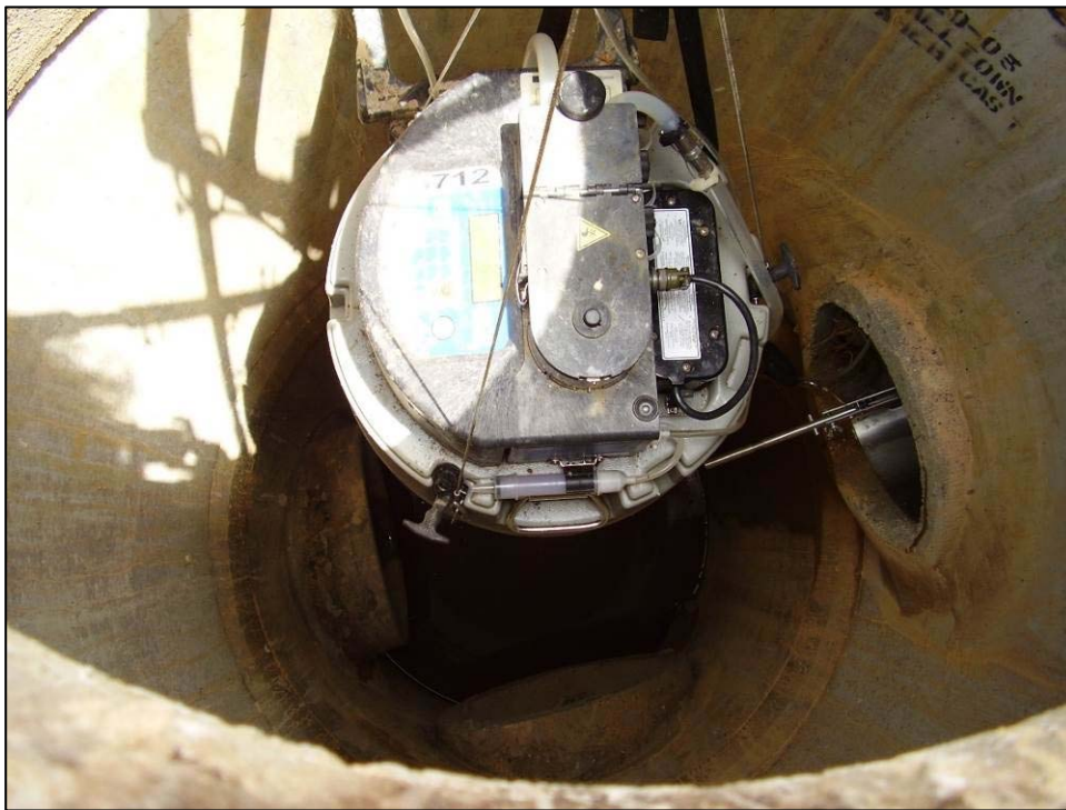
Automated sampler placed in manhole using hanger and spring ring
